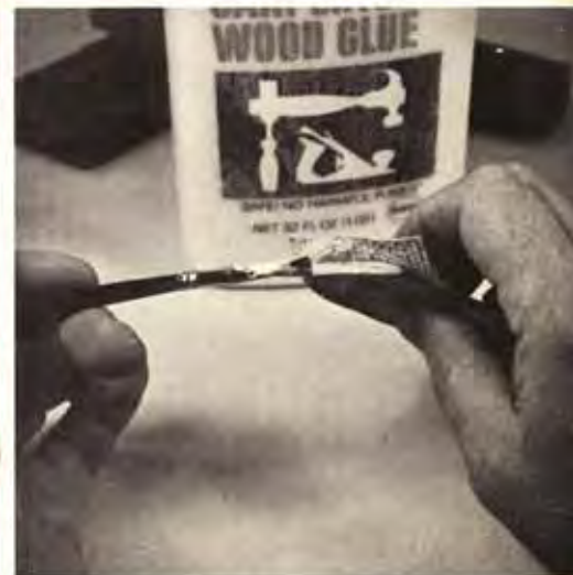
Glue is applied to the top edge and bevel to hold down the loose flap.
